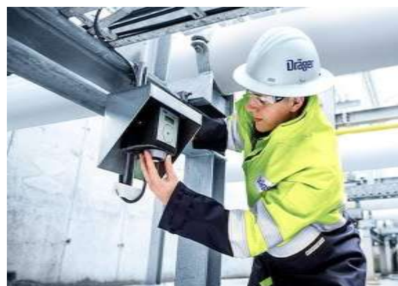
Figure 4: An engineer working on a gas a fixed gas detector [7]
