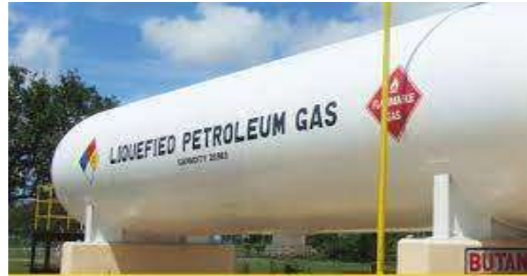
Figure 5: Liquefied Petroleum Gas Tank [13]
