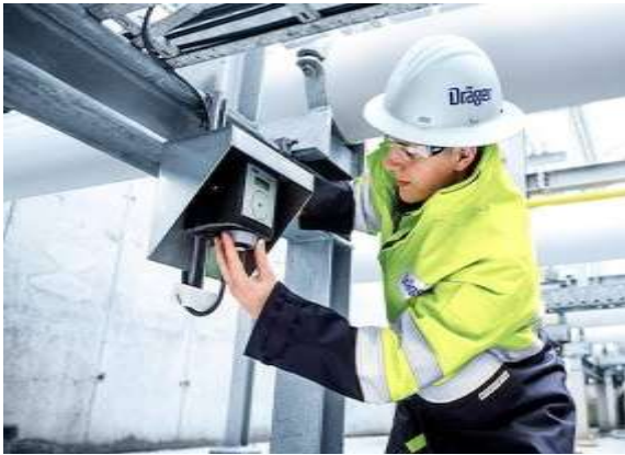
Figure 4: An engineer working on a gas a fixed gas detector [7]
